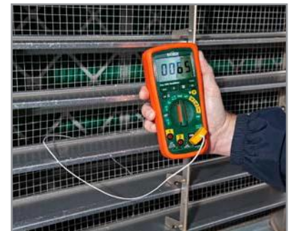
Verify Temperature output on HVAC units using Model EX355
